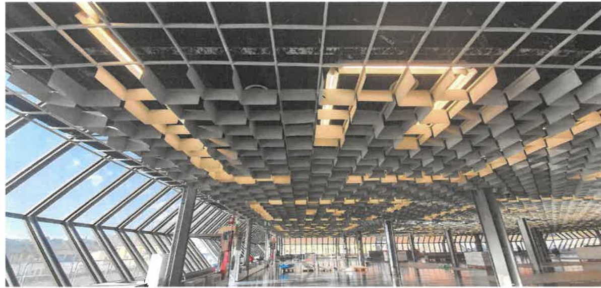
APPENDAGES ARE NOT ALLOWED TO THE FALSE CEILINGS
